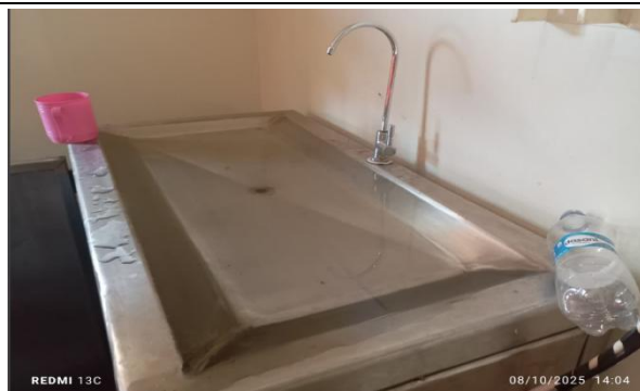
Public drinking water point at the Kenya OSBP
