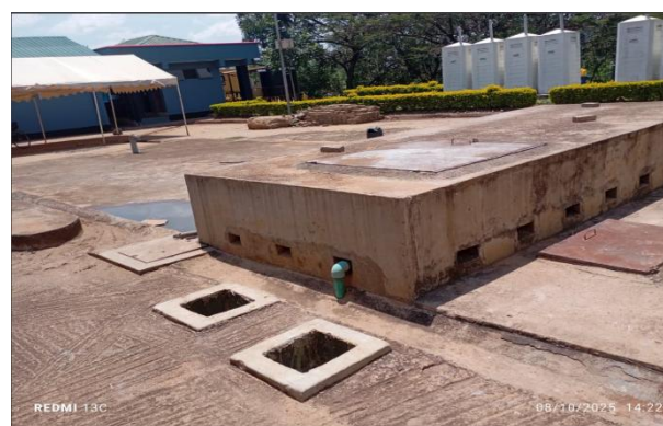
Underground storage tank for rainfall harvesting
