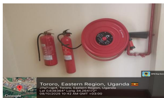
Fire extinguishers installed on site for fire safety
