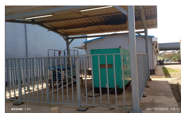
Standby Generator on site.
