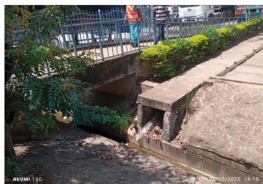
Drainage system onsite
