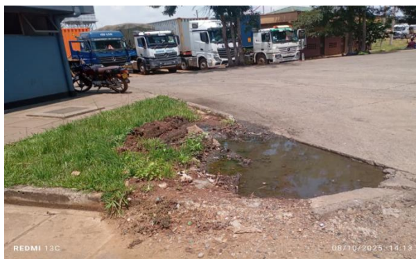
Stagnated water within the compound as a result of limited drainage channels
