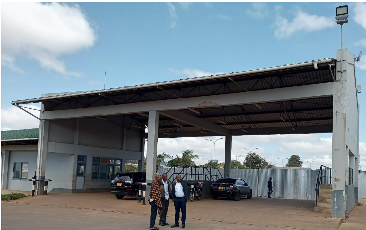
Truck verification bay with no platform for easy verification. The bay has inadequate clearing height for trucks
